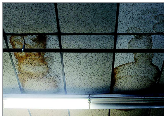
Water stains mark the ceiling tiles in the garage of the Columbia Fire Department's Station 4 on July 7.
