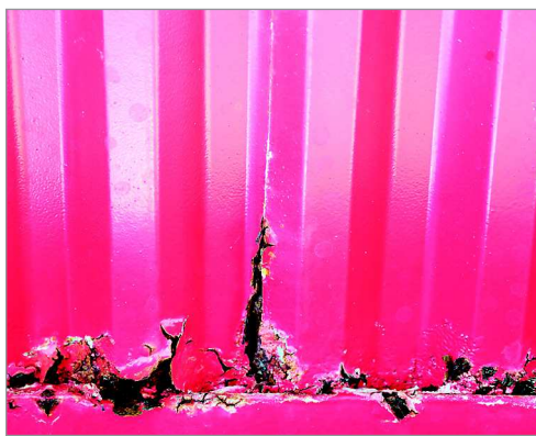
Rust eats away at the tower of the metal ceiling on July 14.
