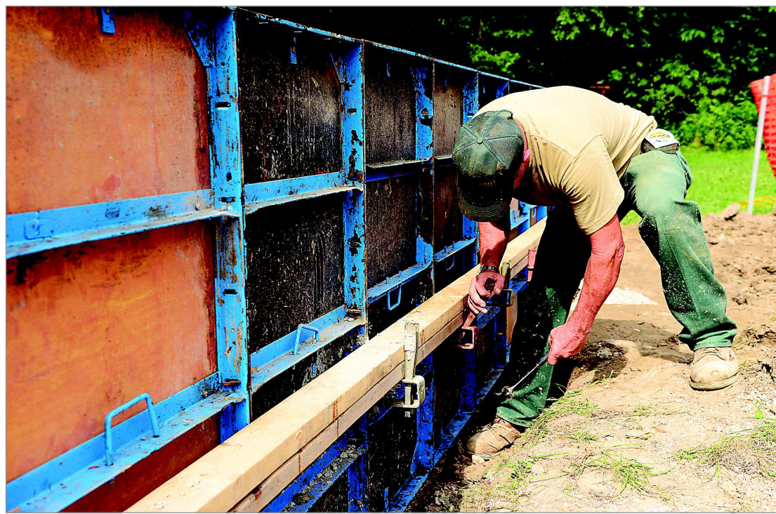
A concrete form keeps the shape of part of the platform being built Wednesday at the entrance to Devil's Icebox Trail in Rock Bridge Memorial State Park. Missouri Department of Natural Resources construction manager Mike Henson said the new entry will include steps leading to a concrete platform, wheelchair ramp, three benches and an information station about the trail and attractions within that section of the park. Weather permitting, the crew hopes to have the project finished by July 31, Henson said.
