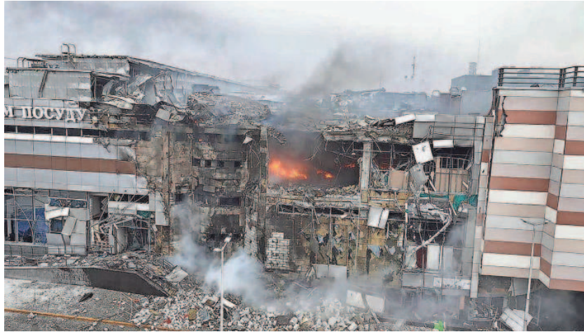
In this photo provided by the Ukrainian Emergency Service, firefighters work in ruins of a mall damaged in Russia's most massive missile attack in Dnipro, Ukraine, Friday, Dec. 29, 2023. UKRAINIAN EMERGENCY SERVICE VIA AP
