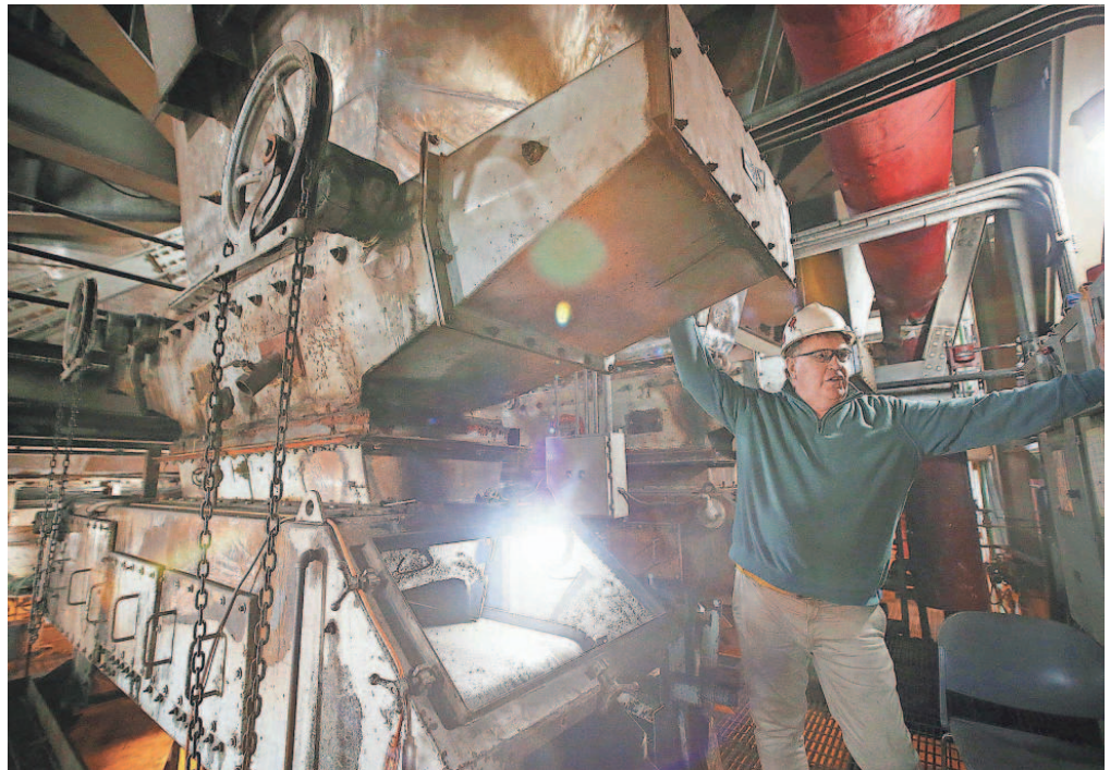
Iowa State University Power Plant operations manager Mike McCurdy explains how the chutes and conveyor belts that brought coal from a silo to a boiler work during a visit on Feb. 28 in Ames.
