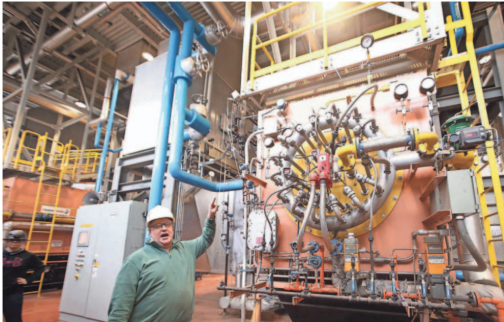
Iowa State University Power Plant operations manager Mike McCurdy explains on Feb. 28, in Ames how natural gas-fired boilers work. Like a giant stove burner, gas enters through the metal ring and burns — but horizontally as a jet of fire — heating up water into high pressure steam.
